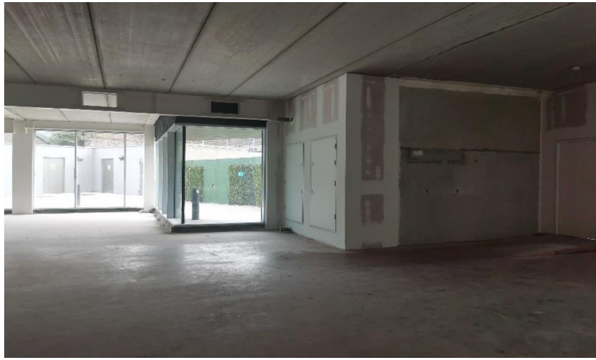
Figure 6.8 Ground floor of Navigation Square building in ‘shell and core’ condition (May 2025)
